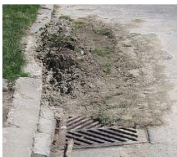
Storm sewer grates that are free of debris are better able to handle stormwater flows and can reduce overland flooding.
